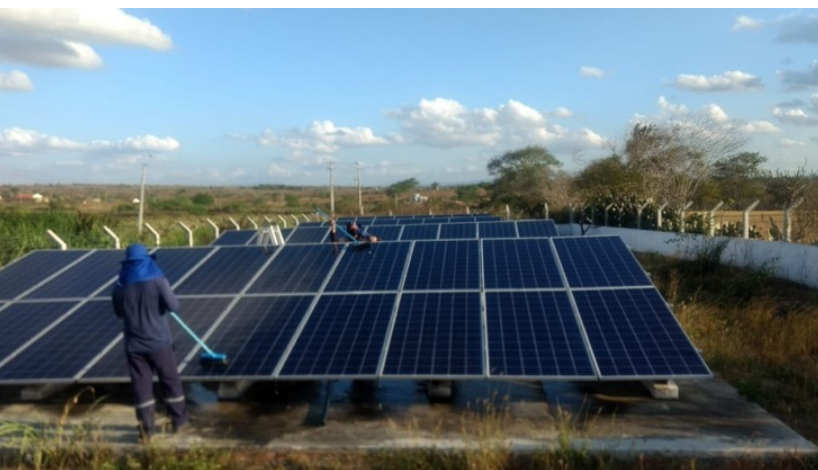
Solar Energy System on-grid in Pernambuco/Brazil (Source: SOL Luções Energia Solar)
